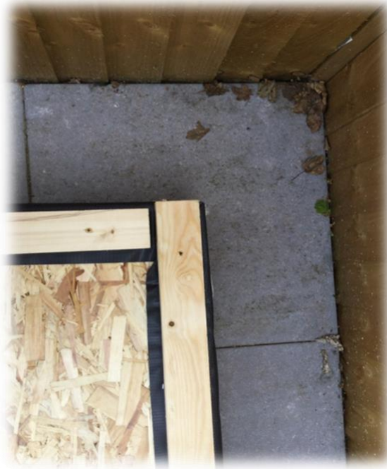
Image above showing the relationship between the side and rear floor plates at back right corner.
